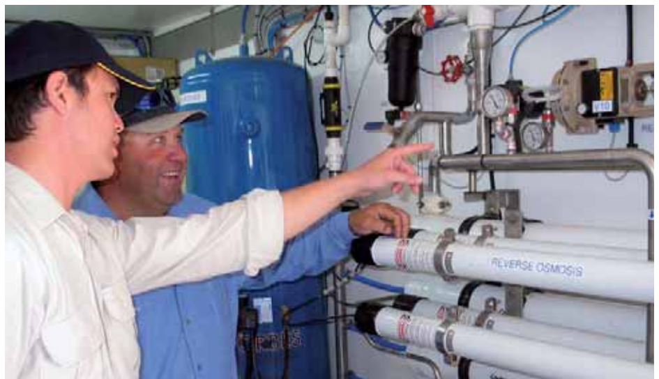
Reverse osmosis treatment plant at Queensland Gas Corporation's coal seam methane facility
